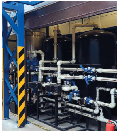
HURIKAN 1000 R - oil sludge disposal
